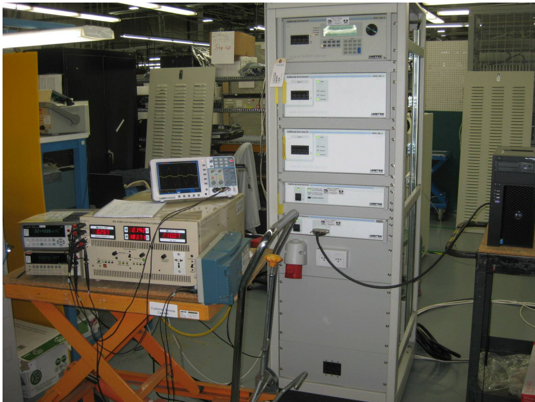
System with new calibration stickers applied.
